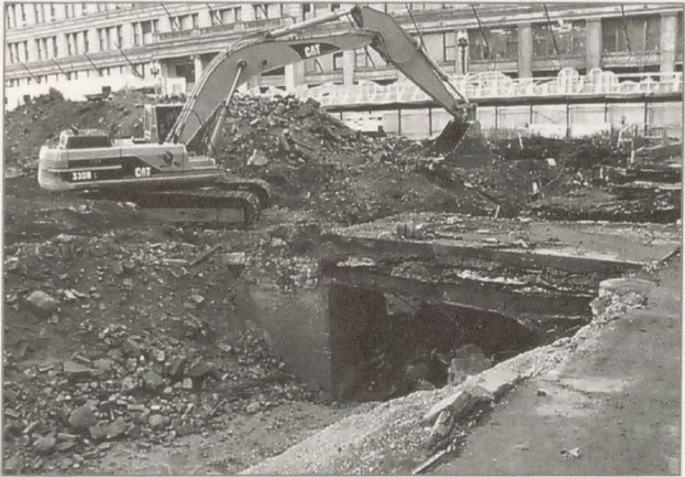
Figure 29. A vaulted sidewalk is visible in the Loop during a construction project.
