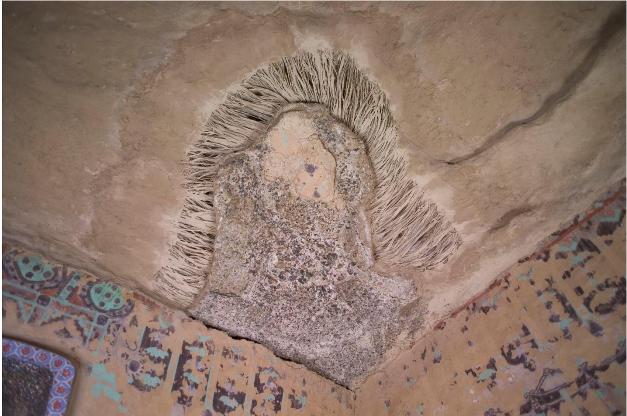
Figure 1-52. Northwest corner of the ceiling slopes in Cave 366 showing mural remains on the rock mass. Photo courtesy of the Dunhuang Academy.
