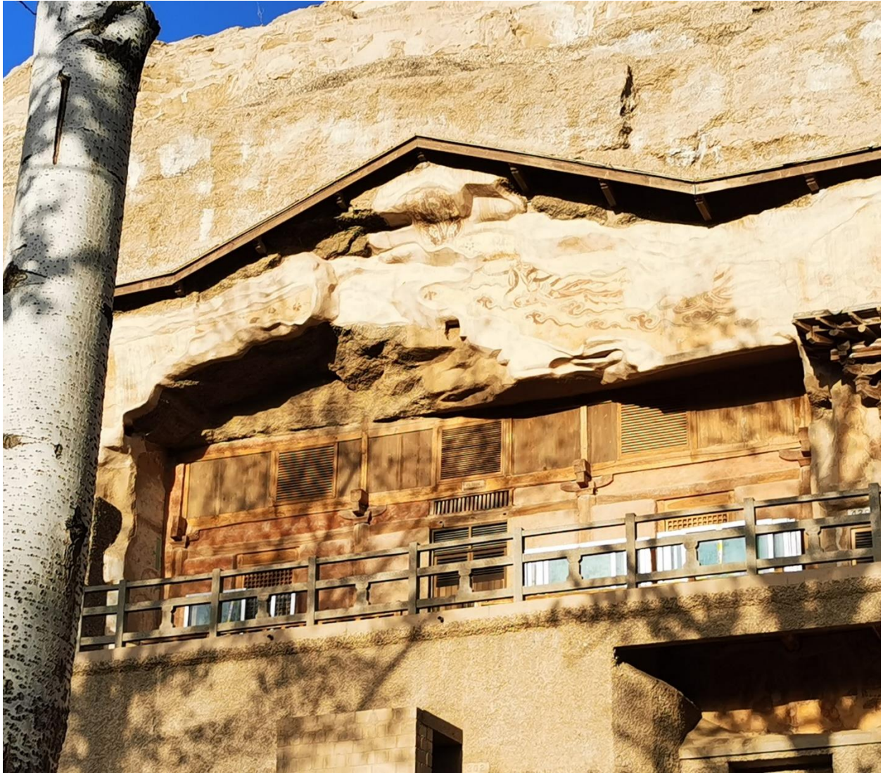
Figure 4-35. The timber-structured façade and open-air mural of Mogao Cave 428. A Qing or modern reconstruction with old timber members from the tenth century. Photo by author.
