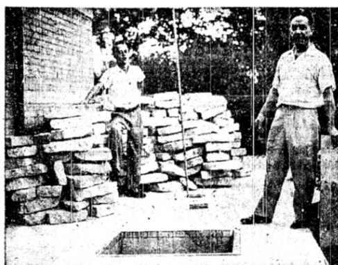
Michael Markel, Hammond engineer, and son Kurt, 16, stand atop roof of steel and concrete bomb shelter they are building next to garage in back yard. Stones in background will be used for garage addition to cover shelter.
