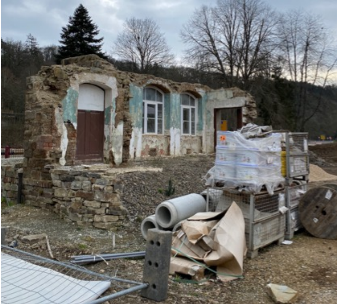
Figure 3. Photograph of a house destroyed by the flash flood in the upper valley municipality of Müsch. Photograph by author.
