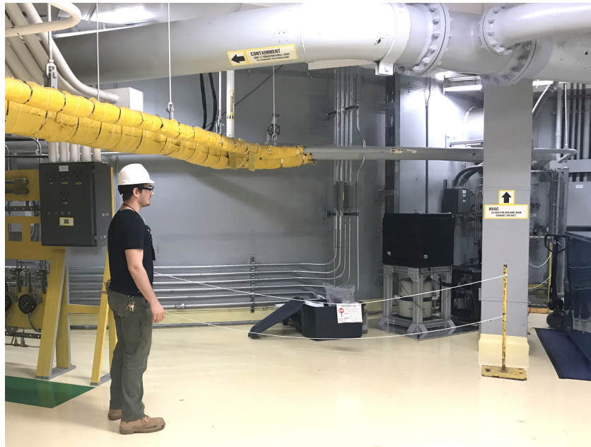
Figure 6.1: Top: Location of the PPC detector within the Mark-I design of the Dresden-II BWR. Figure, adapted from Wikipedia commons, from [191]. Bottom: Author standing next to the installation.
