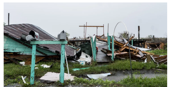
Figure 6: Hurricane Ida decimated the few remaining homes on the island, leaving some structures unrecognizable. Source: Setyawan 2021
