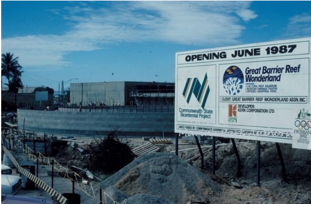
Figure 33. Construction site for the then "Great Barrier Reef Wonderland," now known as Reef HQ, suggesting some of the scale of the enterprise and the considerable public investment involved. (Source: D. Alcock, Great Barrier Reef Marine Park Authority, CC 4.0)
