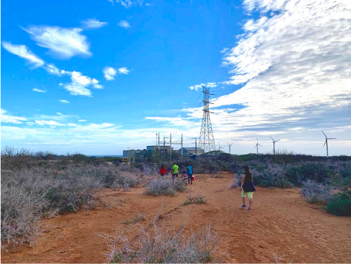
Figure 21. Jepirachi's Electric Substation (Source: Photo by Author)
