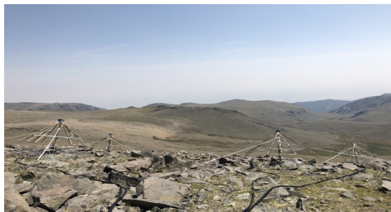
Figure 7.3: View of BEACON prototype from above the mountain ridge. Antennas were camouflaged to minimize environmental impact.
