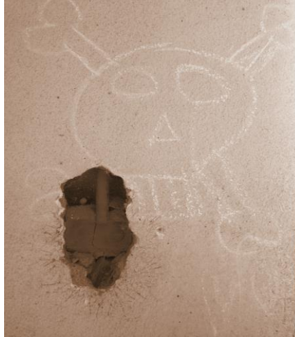
Figure 2. Inside Miguel's daughter's former house, recently invaded by local youth gangs, graffiti comes along with evidence of efforts to strip the house for scrap materials.
