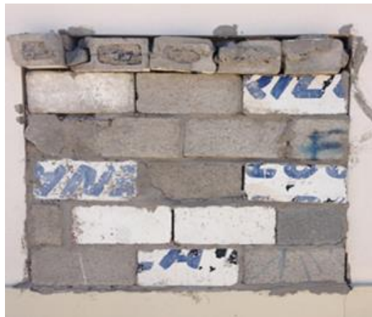
Figure 19. A covered/walled up obra negra (also known as a casa tapada ) owned by Provive, in Riberas del Bravo , 2016.
