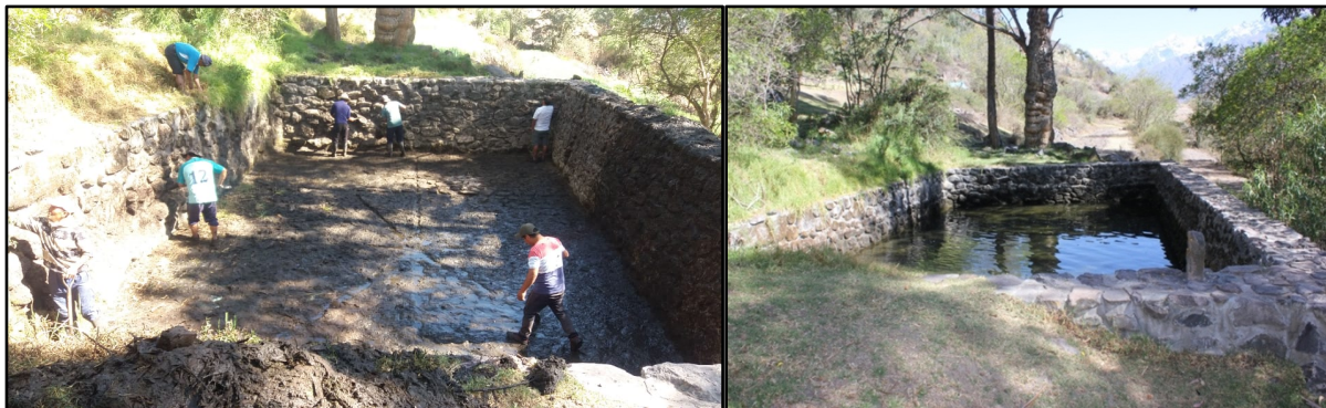
Figure 5-1: One of the two reservoirs at Muyupata, at left partially full of water during the dry season, at right, emptied for cleaning, which is required between one and three times a year depending on sediment accumulation. Note the pile of sediment at the front of the frame of the right-hand photo – Members of the Asociación de Productores Agrícolas de Simapuqio report removing up to several centimeters at each cleaning. Left photo by the author, right photo courtesy of Jose Rodriguez. Note wild plants flourishing around the reservoir due to spillover of water.
