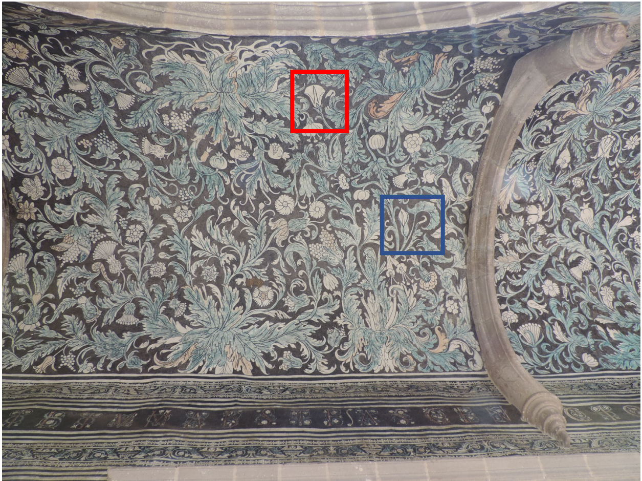
Figure 3.16. Vault, lower cloister walkway. The philodendron is in the blue box and the morning glory is in the red box. San Salvador, Malinalco, ca. 1571. Photo by author.
