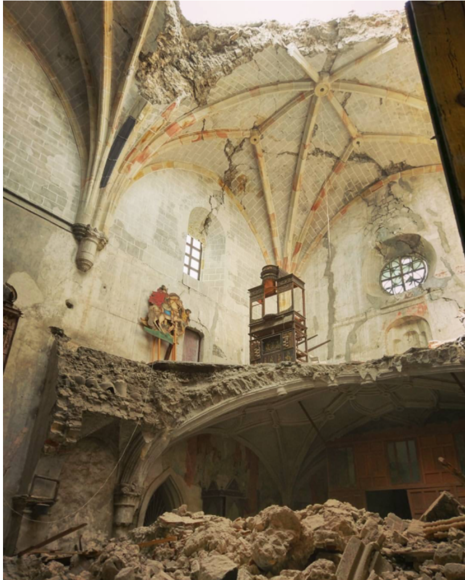
Figure 3.8. Collapsed vault and choir loft of the church. San Martín, Huaquechula. September 2017. Photo in the public domain.
