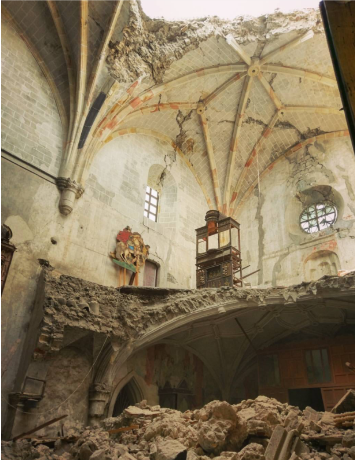
Figure 5.7. Collapsed choir loft. Church of San Martín de Tours, Huaquechula, ca. 1569. 25 September 2017. Image in the public domain.
