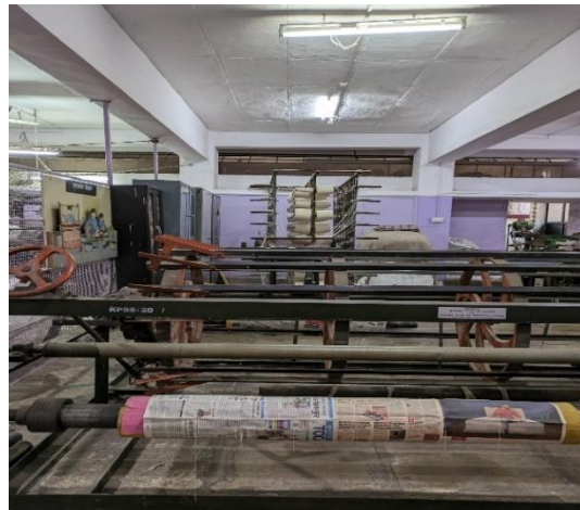
Image 4: Power loom room at Sankalp workshop with white ceilings and a bright tube light for illumination.
