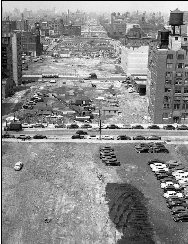
Figure 8: Congress Expressway land clearance in 1951, looking west from the Main Post Office. Congress Expressway Construction , by William Deluga, from the Chicago History Museum. 93
