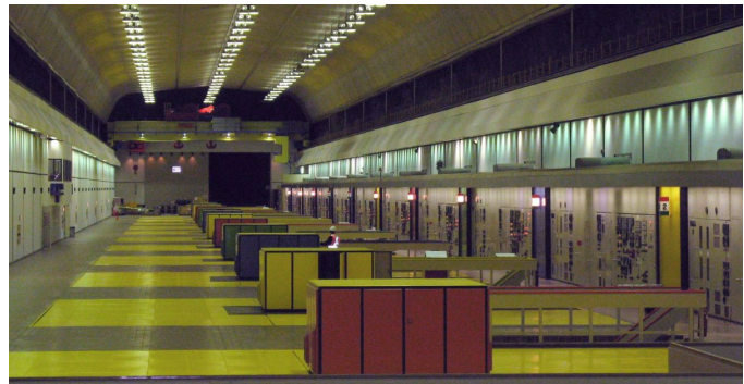
Image 32: Powerhouse turbine hall Interior of Churchill Falls Powerhouse by Kevin Bisset
