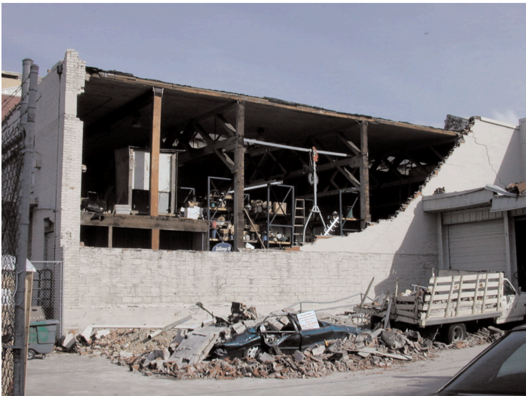
Figure 6. “Collapsed hollow-clay tile wall at URM building located along Utah Ave. S in South Seattle” (State of Oregon Department of Geology and Mineral Studies, 2001, p. 6)
