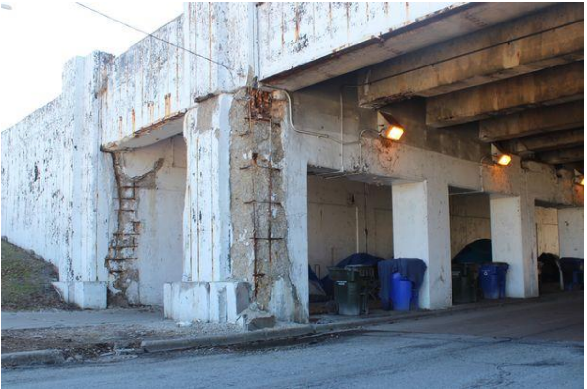
Figure 3. That the Lawrence viaduct was declared structurally deficient in 2017 came as no surprise to anyone who had walked near it. (Picture by Josh McGhee for DNAinfo)
