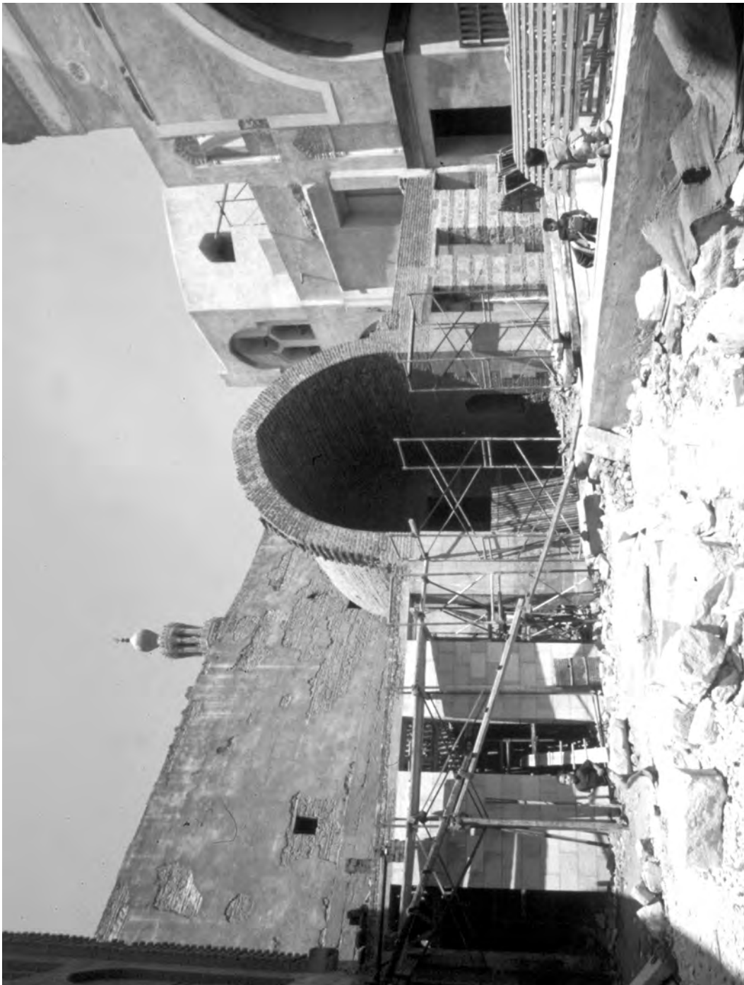
Fig. 13. Madrasah of al-Nāṣir Muḥammad, northern iwān during reconstruction in front of the mausoleum, 1987 (Speiser)
